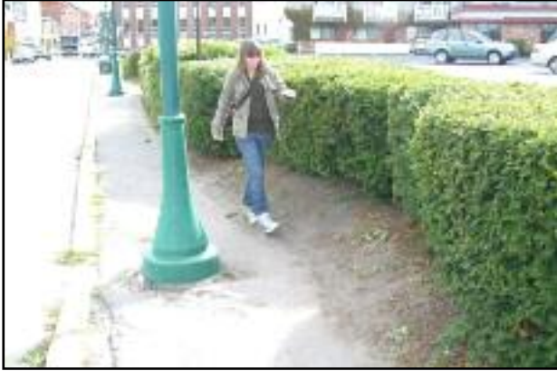
Sidewalk conditions between Summer Street north to North Main Street are often dangerous and not ADA compliant. In this photo the placement of light posts and the large bases forces pedestrians to walk off the sidewalk. The vegetation has been trimmed back to accommodate pedestrian movement.
